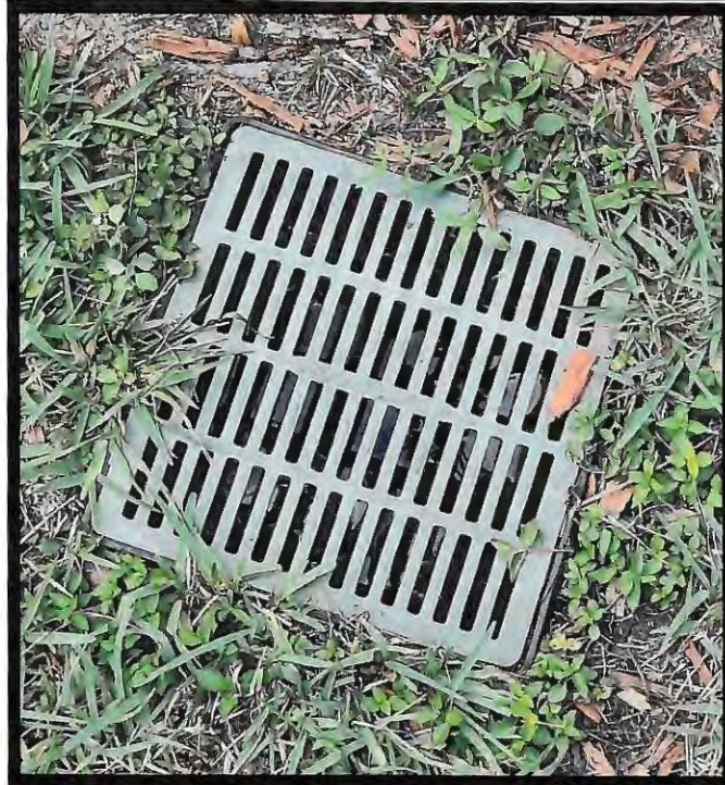
Figure 1: Evidence of bubble-up structures holding water in dry conditions
