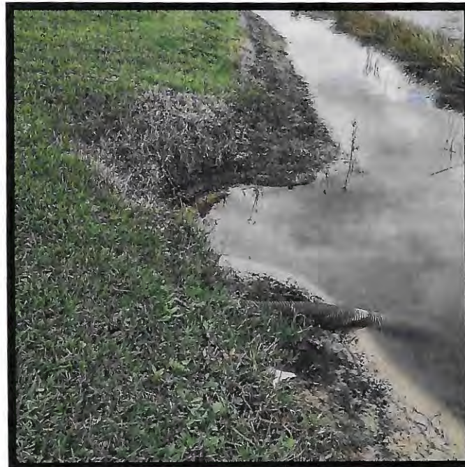
Figure 3: Northeastern lake bank erosion – shared neighbor utilizing underground pipe for roof drains
