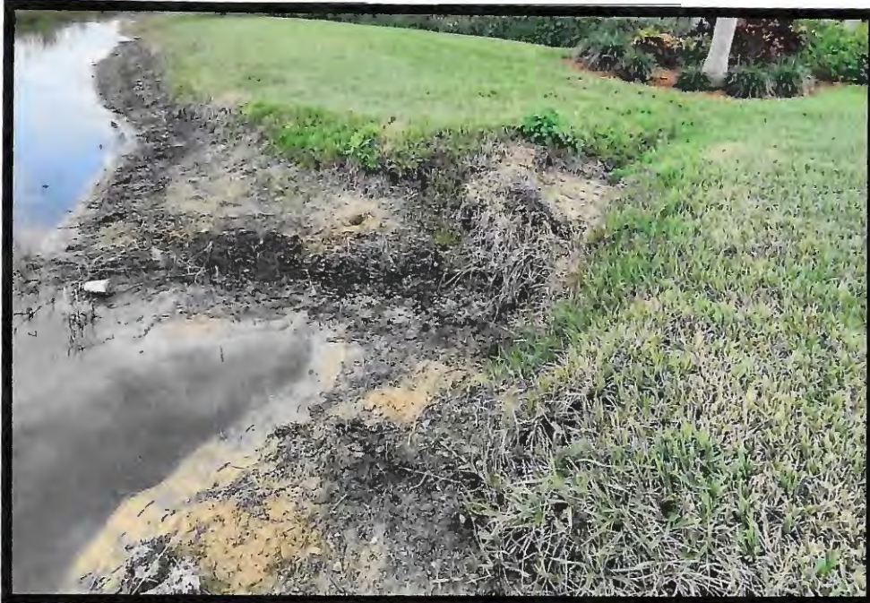
Figure 4: Northwestern lake bank erosion – shared neighbor contributing sheet flow via roof drains
